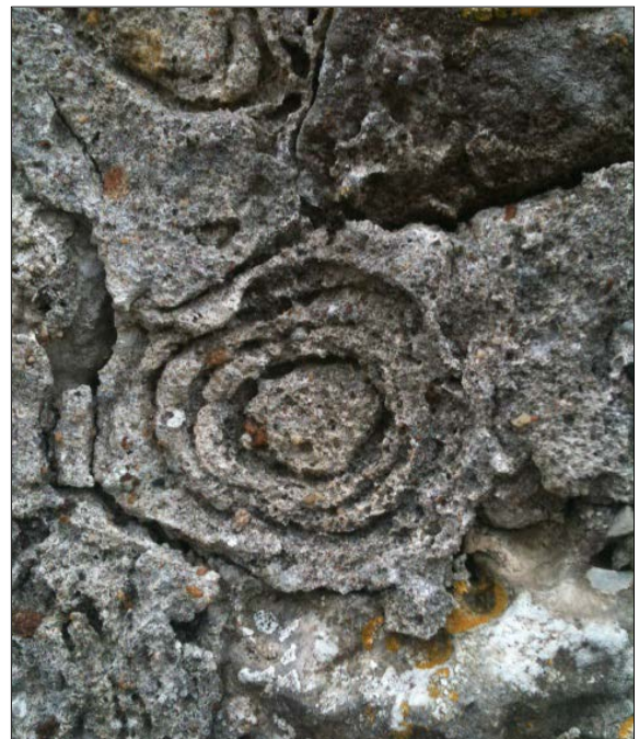
Unexplained marks in lime mortar
